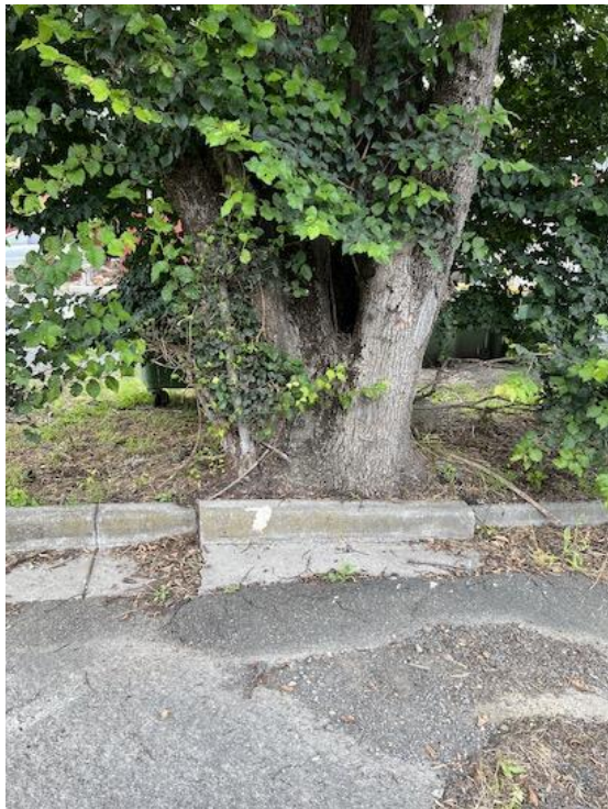
Tree 2 trunk roots cracking curbing & bitumen
